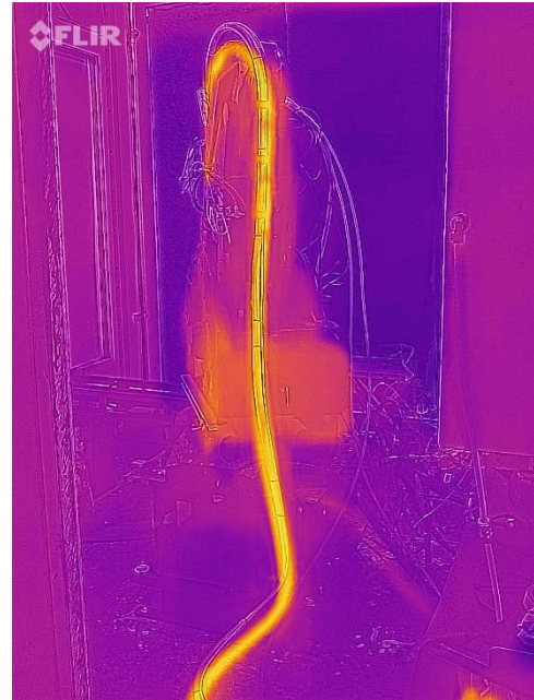
Figure 10: Thermal Scan Showing Control to Point of Dispense
